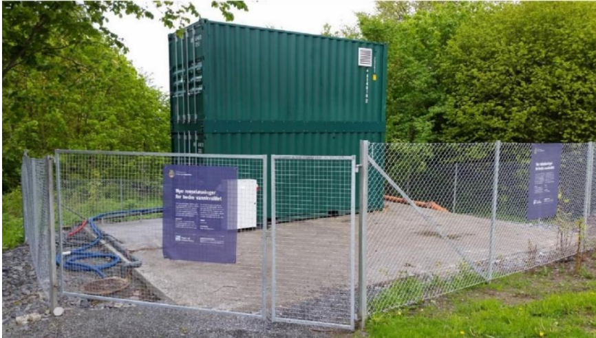
Figure 7 Container type HRF demonstration plant
